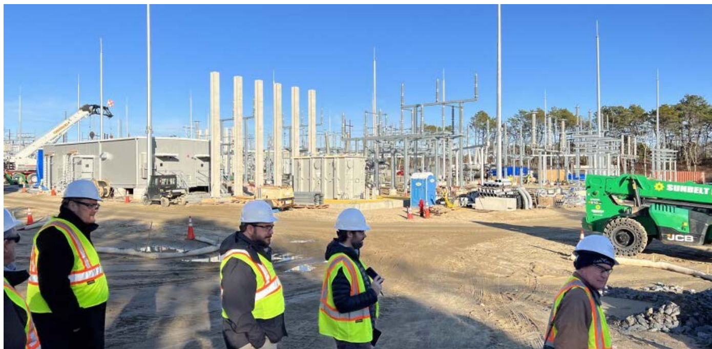
FIGURE 8: Substation for Vineyard Wind Cables
