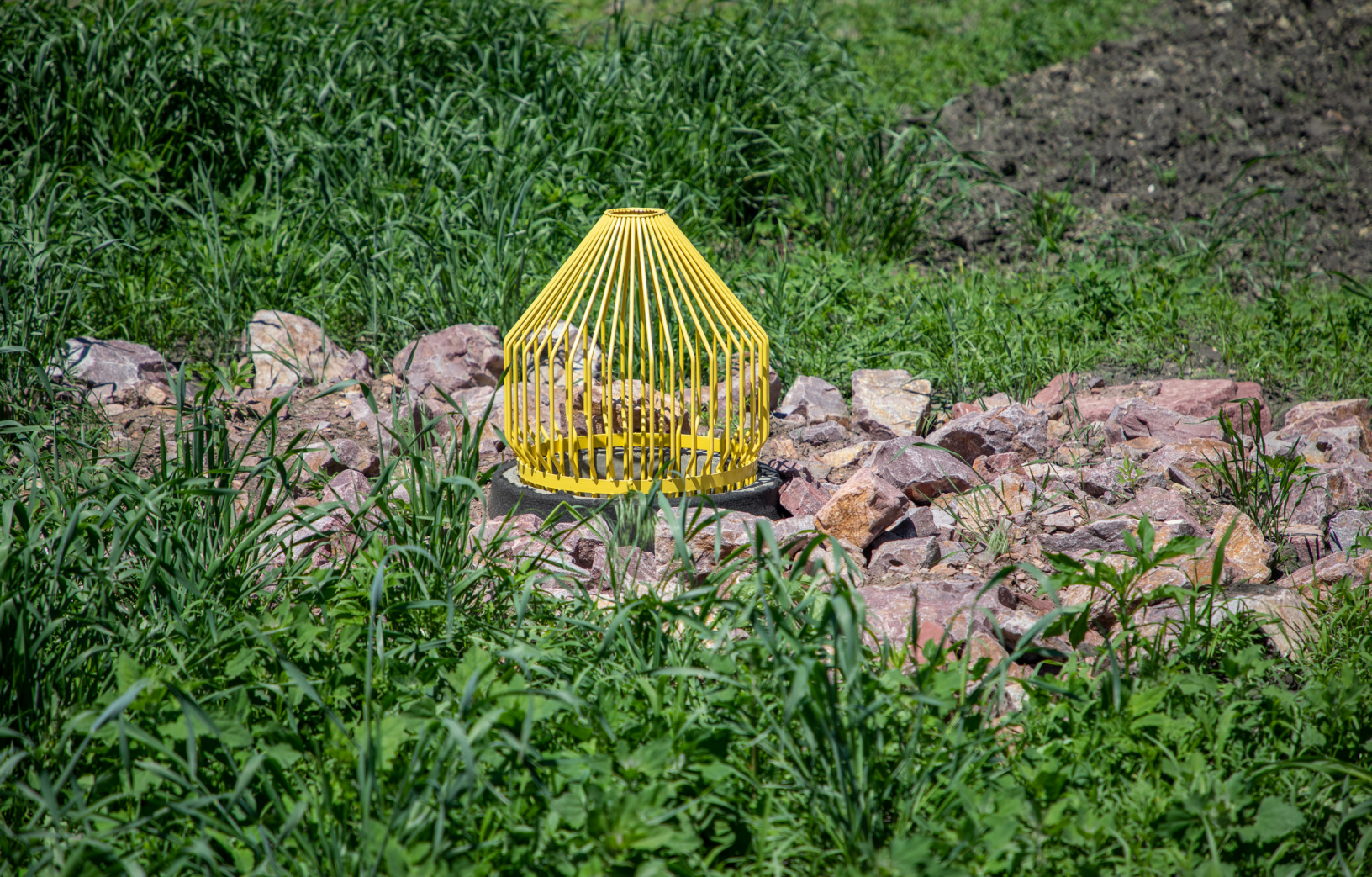
Figure 15: A surface intake into a drainage system with a bar guard to prevent debris from entering the system.
